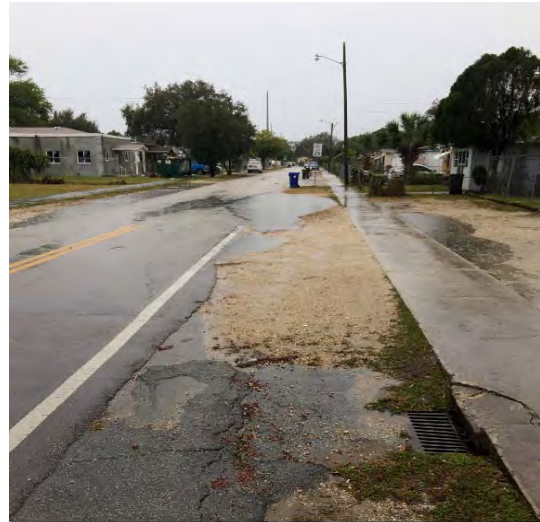
NW 15th Way between NW 5th Street and NW 6th Street on February 22, 2017. Example of poorly graded/paved swales.
