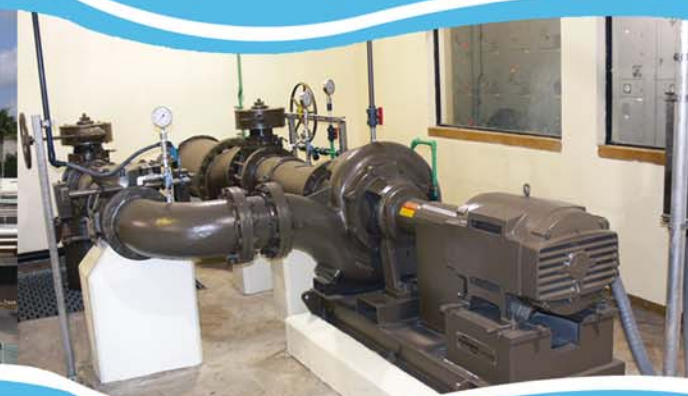
Return Sludge Pump Station
