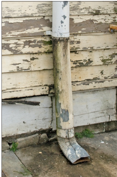
The downspout is discharging immediately adjacent to the building onto a concrete surface. The bottom of the downspout is crushed, likely resulting in clogging. The storm water splashing onto the concrete surface can saturate the wood wall and masonry foundation. The wood adjacent to the downspout exhibits visible deterioration.
