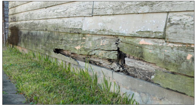
Wood located on or next to a masonry foundation is more likely to absorb moisture and rot, as well as attract termites and pests.
