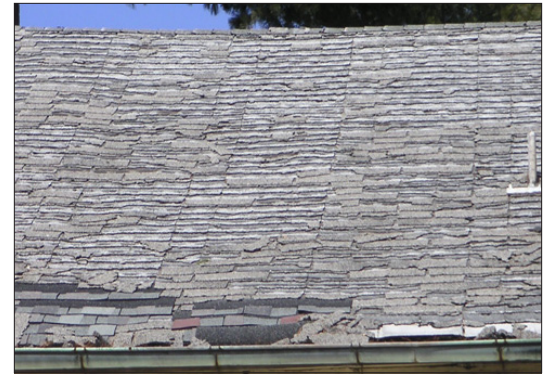
The bow at the top of the roof suggests a structural problem that should be reviewed by a professional. The mineral granules of the asphalt shingles have worn away and shingles are broken and patching evident. The roof should be replaced after structural repairs are completed.
