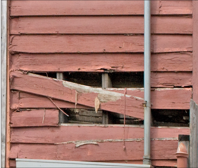
Portions of the siding are missing or dislodged, exposing the interior wall framing and interior plaster lath to the elements. Openings in the wall can allow moisture penetration and result in rotting of structural framing.
