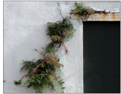
The cracks in the stucco are supporting plant growth, suggesting high moisture in the wall. Also note the rusting lintel above the door.
