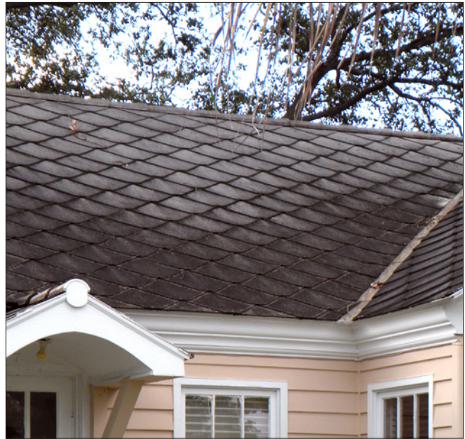
Although asbestos roofing was available in a number of different patterns, diamond-shaped shingles, such as those illustrated above, were by far the most common.
