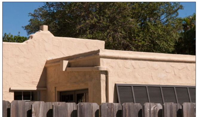
The downspout has been painted to match the color of the wall, reducing its visual prominence.
