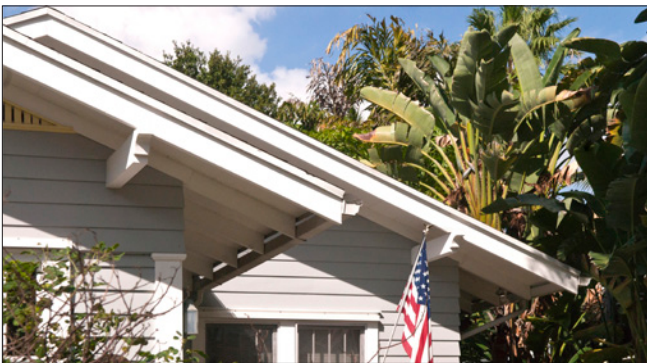
The extended eaves have exposed rafter tails and jigsaw-cut outriggers providing support.
