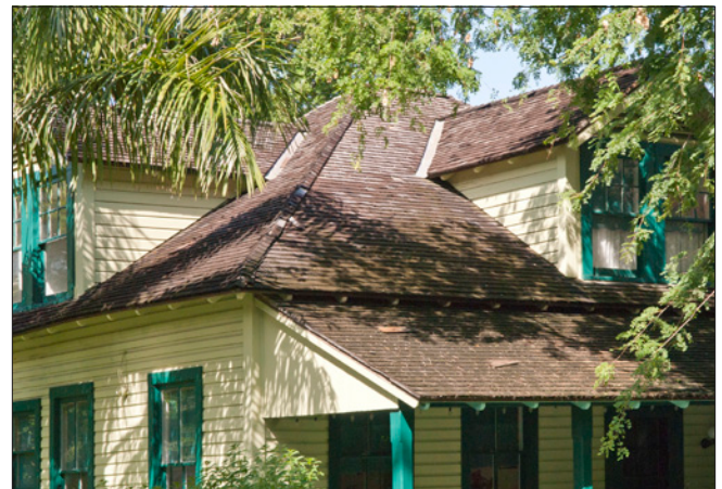
Wood shingle roofs can be found on some of Fort Lauderdale’s oldest homes.
