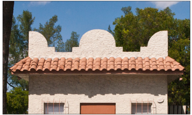
Flat roof are often hidden from view. In this case, a decorative parapet conceals the flat roof beyond. A terra cotta pent roof, located below the parapet, circles the building.
