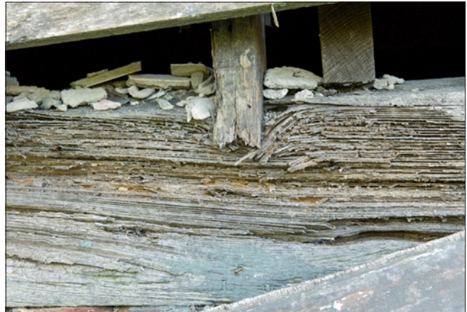
Termites have eaten the wood along the grain, weakening the wood sill. The pressure from the wood studs crushed the top of the weakened wood sill causing structural problems at the wall above.
