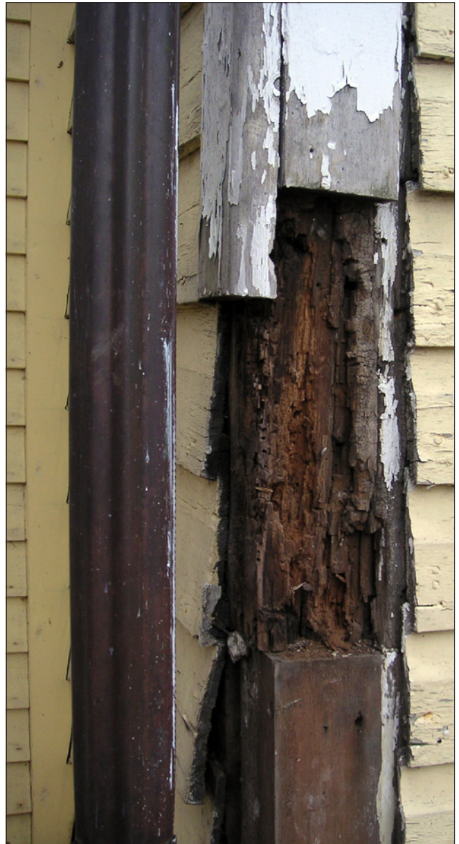
The vertical wood corner boards were removed adjacent to the downspout exposing the structural wood post. Additional exploration revealed that there was significant rot of the post that extended deep into the thickness of the wood, compromising the structural capacity. It is likely that a persistent leak at the juncture of the roof gutter and downspout made the situation much worse.
