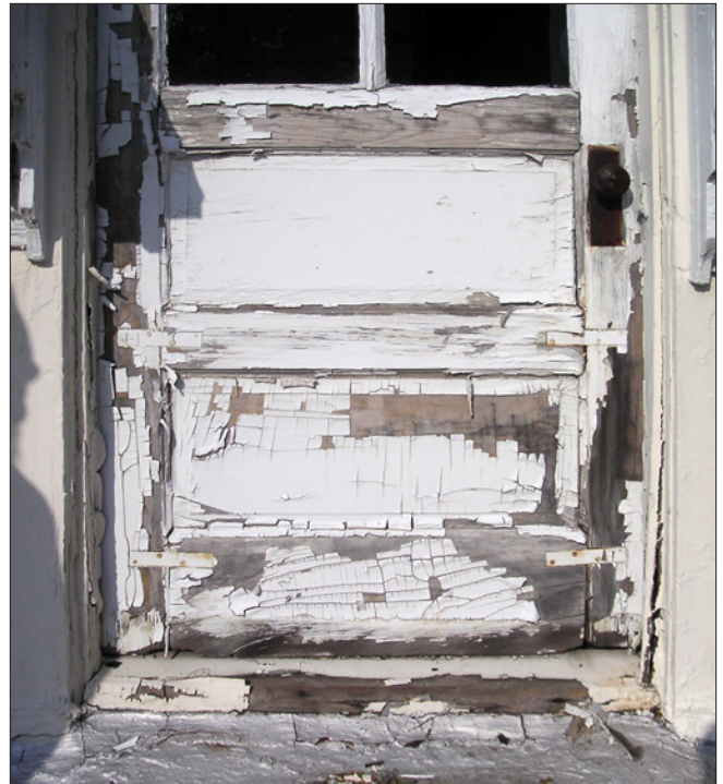
The paint on this door has alligatored, and severe cracking is visible. Removal of paint down to bare wood and proper door repair are recommended prior to repainting.
