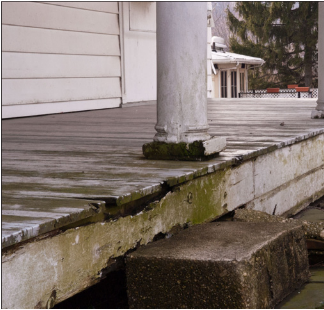
Porches, steps and other areas where the woodwork is laid horizontally or located close to the ground are often first to deteriorate. Ongoing exposure to moisture can lead to rot of the column bases, porch deck and apron.
