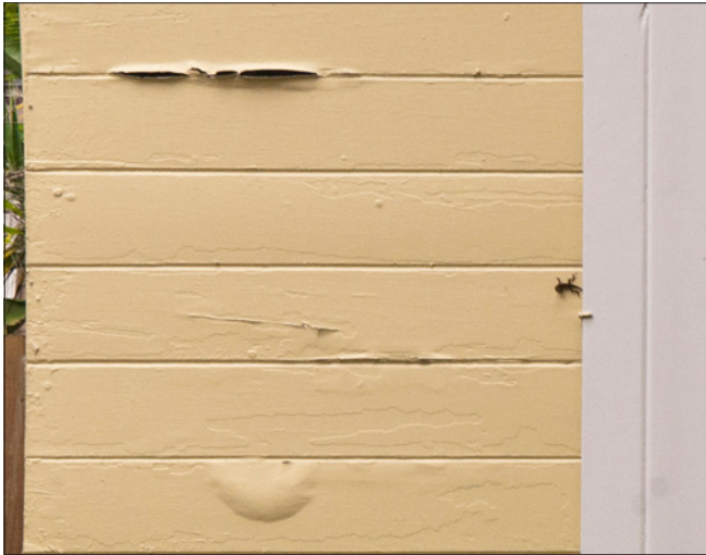
The blistering and peeling paint are a possible indication of moisture problems.
