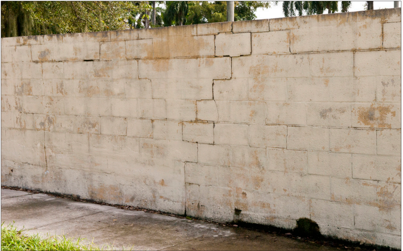
Garden walls are more likely to have problems since they are exposed to the weather on both sides and are not necessarily as well maintained as building walls. This example exhibits open joints, displaced concrete block, peeling paint and staining from moisture along the sidewalk.
