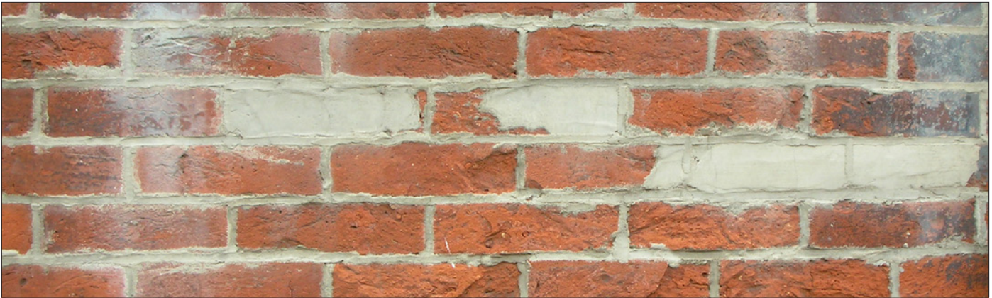
The rough texture and uneven surface of this brick suggest that an aggressive cleaning method was used. Stucco patches replace bricks and efflorescence, a powdery white substance, can be seen on the surface.
