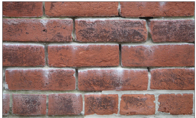
The mortar joints between bricks has deteriorated, particularly at the vertical joints, increasing the potential for mortar infiltration. The area at the lower right corner of the photograph has been recently repointed and mortar has been smeared over the surface of the brick rather than tooled. To maintain the historic appearance, it is recommended that the replacement mortar match the historic in appearance, color, texture, hardness and joint profile.
