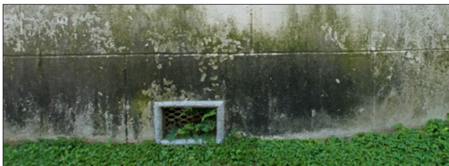
Algae growth is an indication of a moisture problem.
