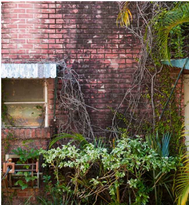
The dark staining and vine growth on this brick wall surface is likely due to moisture in the wall. Removal of the vines and shrubs immediately adjacent to the building will increase ventilation of the wall surface and allow it to dry-out. The wall can then be cleaned to remove the dark staining.
