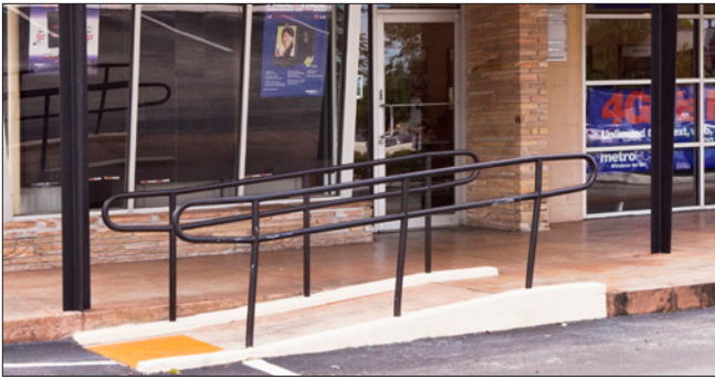
The ramp provides access to the raised landing surrounding the building. The railing is simple and complements the architectural style.
