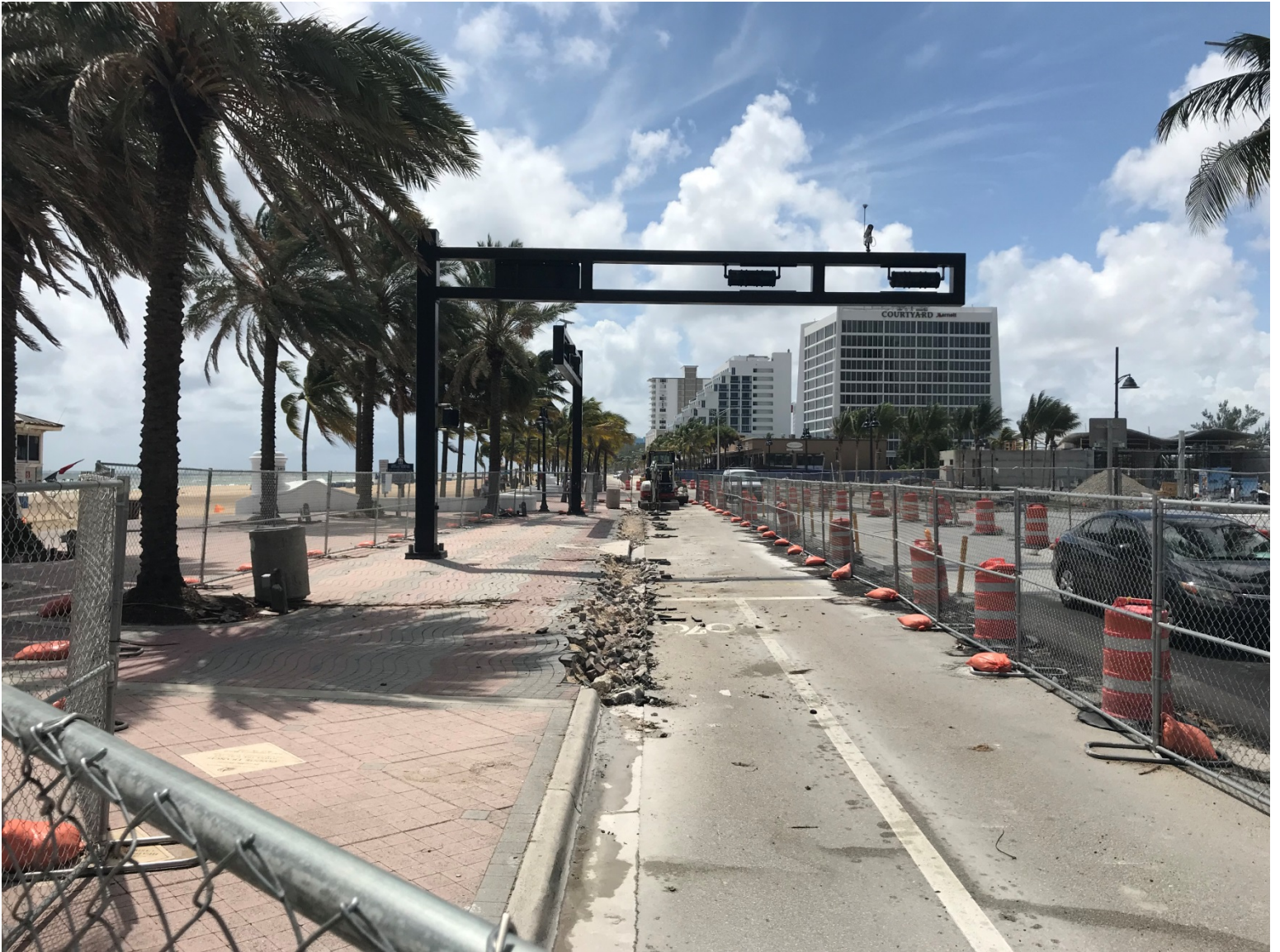
FESTIVAL STREET PROGRESS PHOTO TAKEN ON 9-12-2019 (SR A1A FACING SOUTH – LANE SHIFT HAS OCCURRED AND WORK STARTED ON OUTSIDE LANE)
