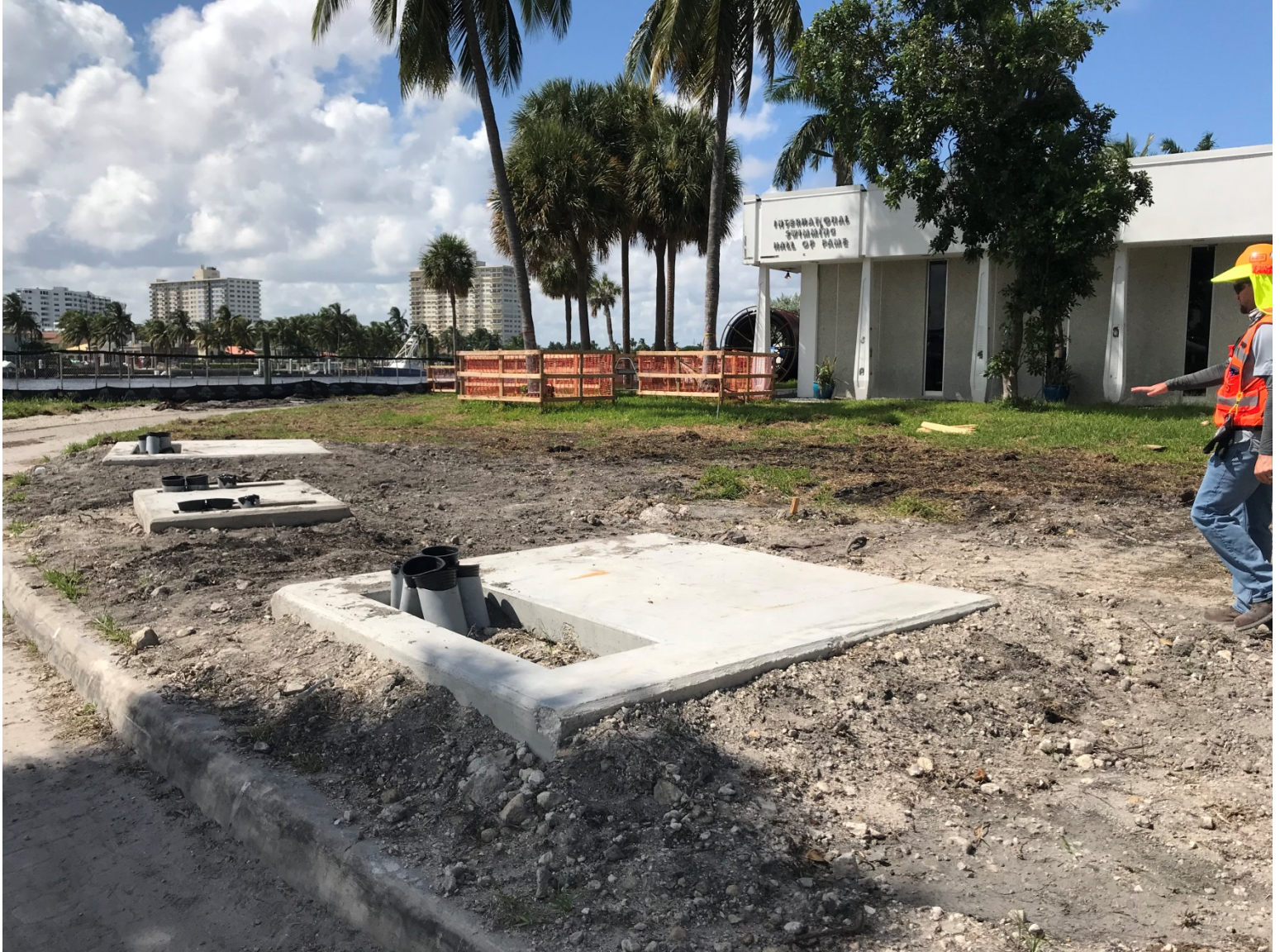
AQUATIC CENTER PHOTO TAKEN ON 9-10-2019 (SOUTH SIDE OF FACILITY – FACING WEST – TRANSFORMER PADS AND CONDUIT INSTALLED)
