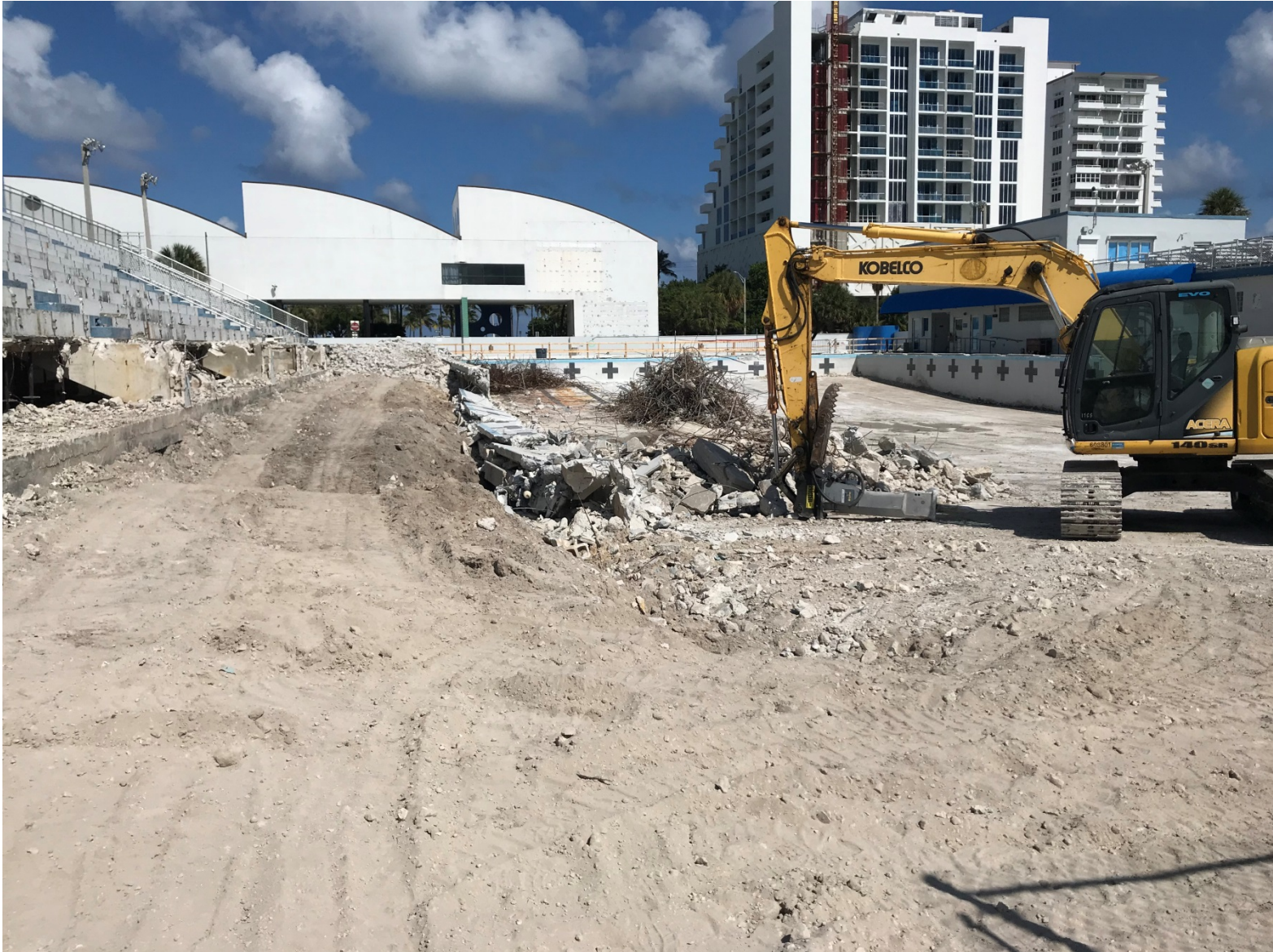
AQUATIC CENTER PHOTO TAKEN ON 9-10-2019 (FACING EAST – COMPETITION POOL AND POOL DECK DEMOLITION)
