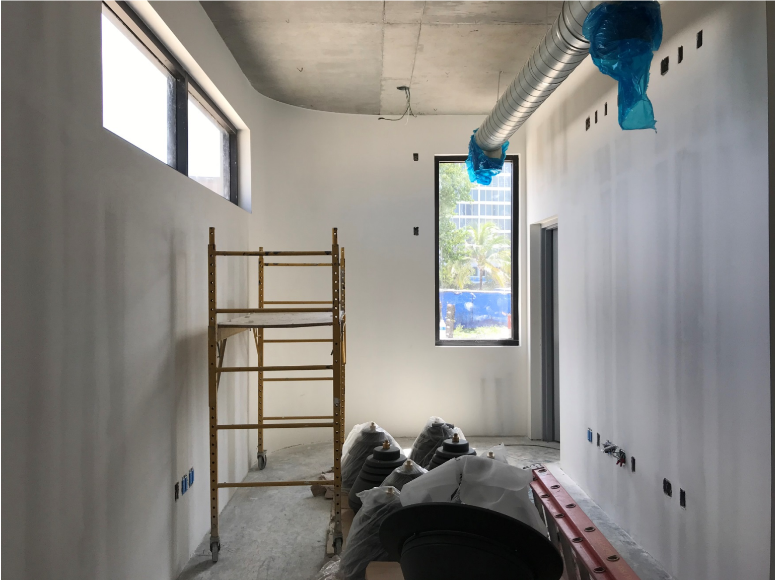
OCEANSIDE PARK PROGRESS PHOTO TAKEN ON 9-11-2019 (INTERIOR OF POLICE SUBSTATION AND VISITOR CENTER)
