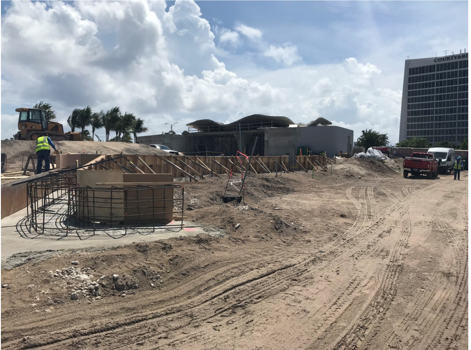
OCEANSIDE PARK PROGRESS PHOTO TAKEN ON 9-12-2019 (CAST-IN-PLACE SITE WALL FORMWORK AND FOUNDATION)
