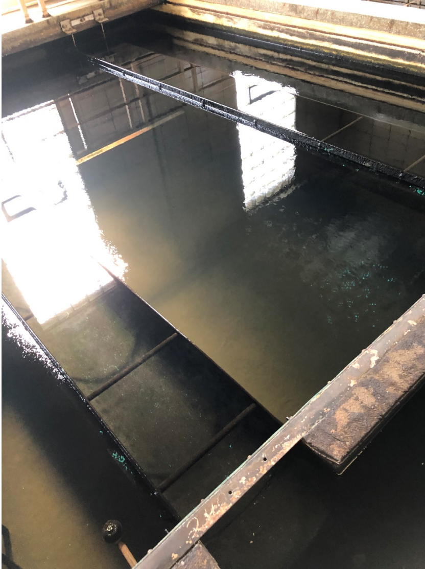
Figure 5.3 6 mgd Aliquippa Municipal Water Authority Concrete Filter Box Ion Exchange System
