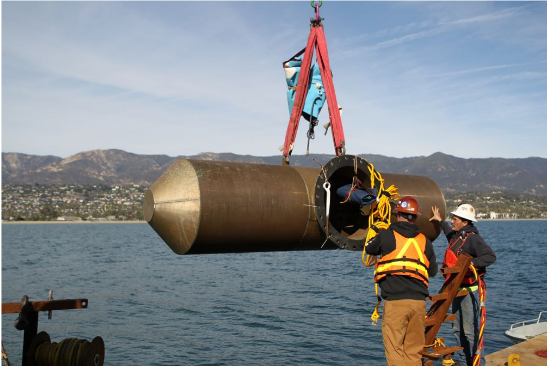
Cylindrical wedge wire intake screens – Santa Barbara, California
