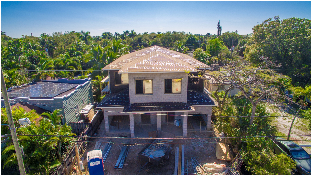
BELOW – 1010 SW 2 nd CT with Horizontal Slider Windows reflecting same metal to glass ratio with pre-untin installation;
