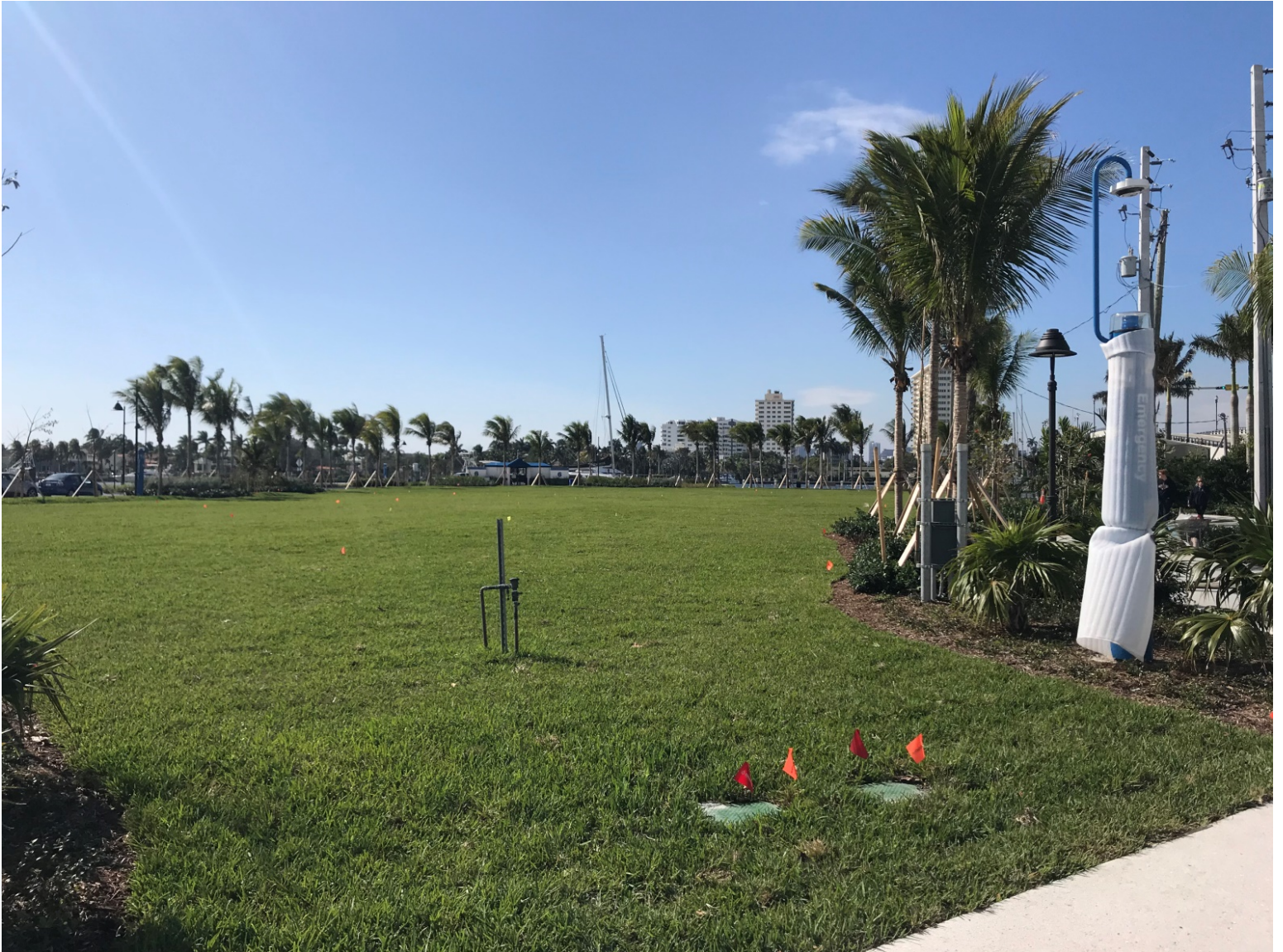
LAS OLAS PROJECT PROGRESS PHOTO 1-22-2020 (SOD INSTALLATION SOUTH OF LAS OLAS BRIDGE)
