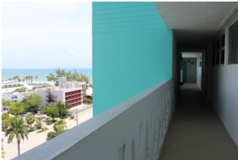
Image 29: Birch Tower, North Façade, Balcony, Looking North-East Photo: Morris Hylton III, April 19, 2019
