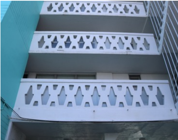
Image 31: Birch Tower, North Façade, Precast Concrete Railings, Looking South and Up Photo: Morris Hylton III, April 19, 2019
