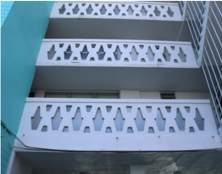
Image 31: Birch Tower, North Façade, Precast Concrete Railings, Looking South and Up Photo: Morris Hylton III, April 19, 2019
