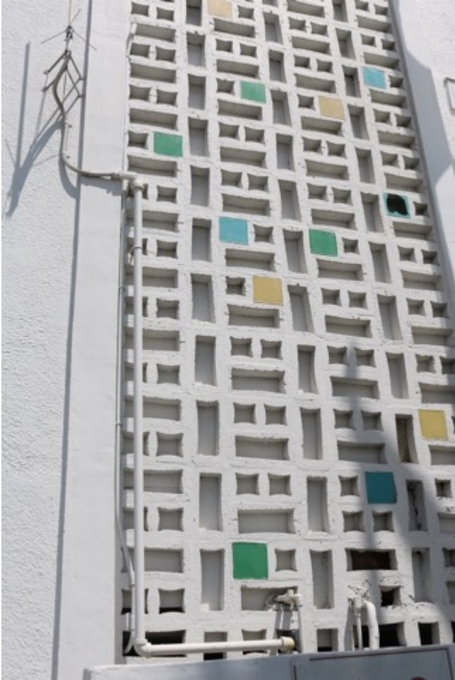
Image 11: Birch House, Ornamental Screen Block, Looking East Photo: Morris Hylton III, April 19, 2019
