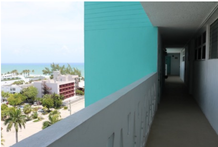
Image 29: Birch Tower, North Façade, Balcony, Looking North- East Photo: Morris Hylton III, April 19, 2019
