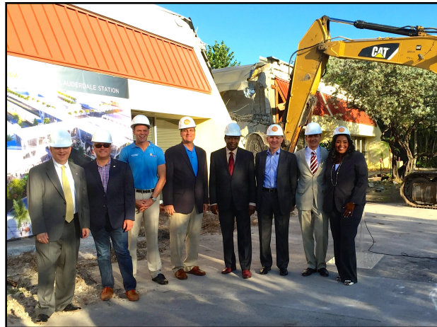
Commissioner Trantalis joins Mayor Jack Seiler and other city and county officials to break ground on the downtown train station for the All Aboard Florida line.
