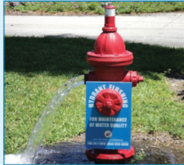
Flushing fire hydrants is a routine part of the free chlorination process.
