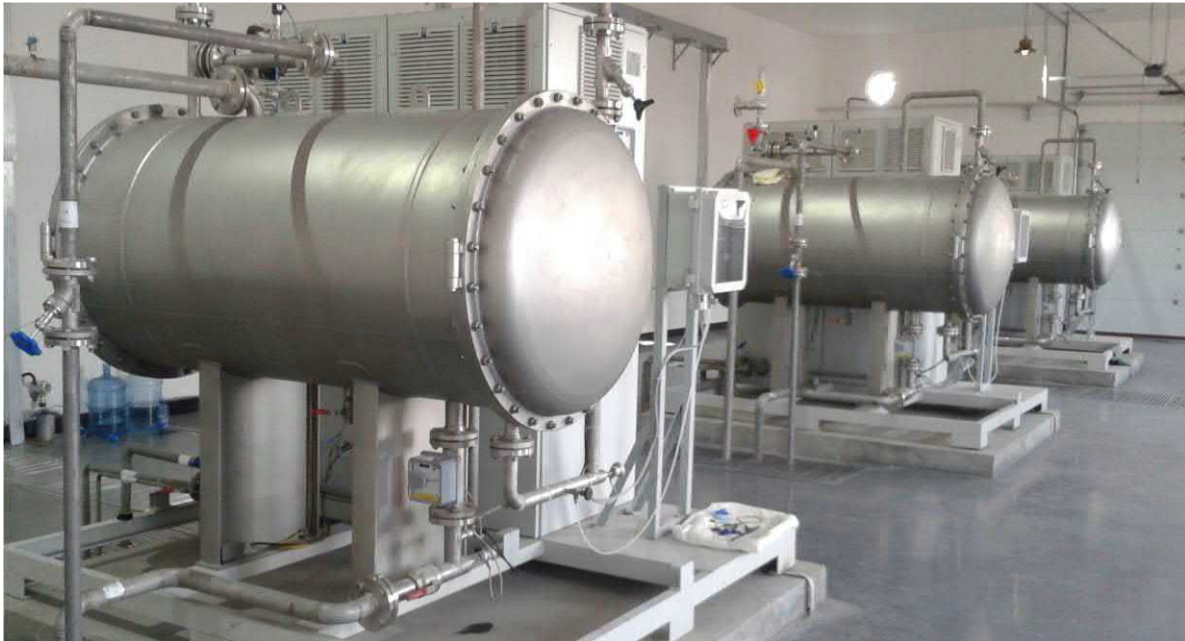
Drinking Water Treatment Plant - 3 x 620 PPD
