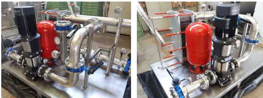
typical close loop cooling system skid
