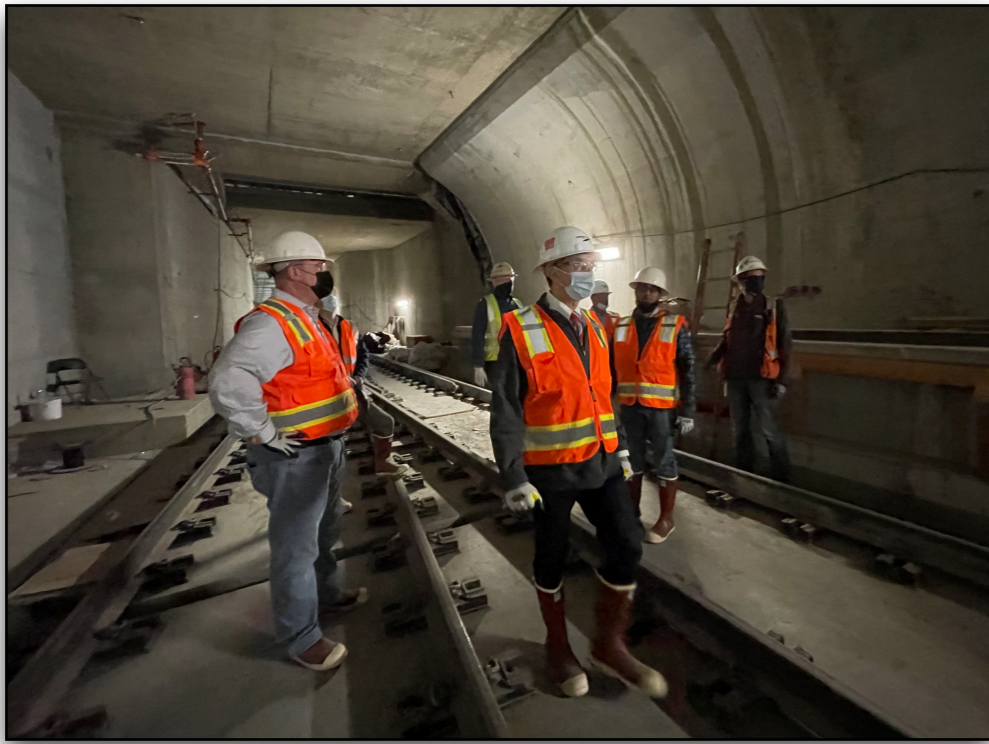
Mayor and city manager inspect Traylor Bros.' work on Los Angeles subway under the La Brea tarpits.
