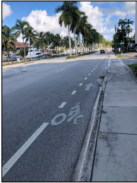
Bicycle Lane - Pavement Marking Faded
