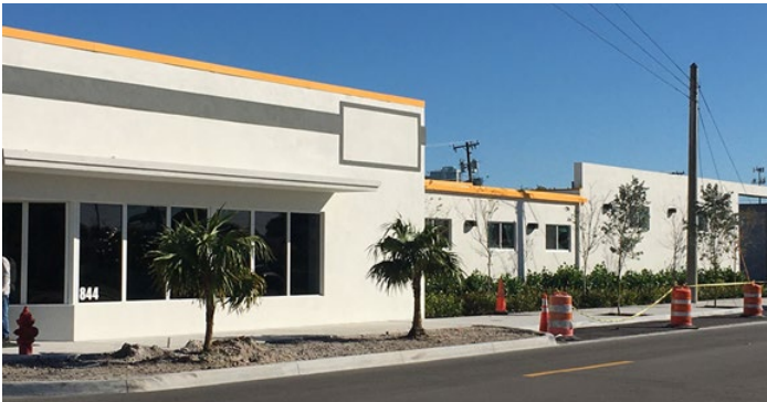
Commencement of renovation and expansion of Hoover Canvas products at 900 NW 9 Avenue
