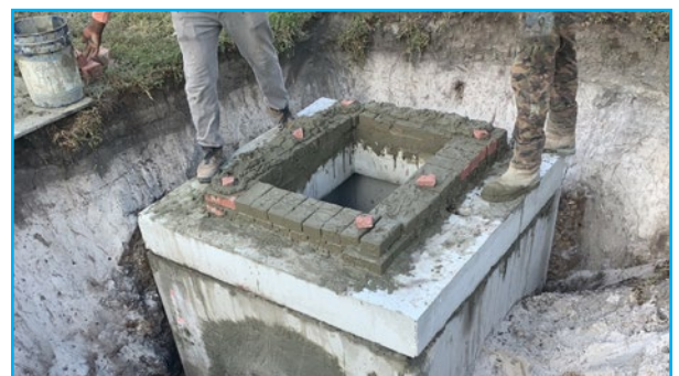
Crews installing a new catch basin that will collect stormwater in Edgewood.
