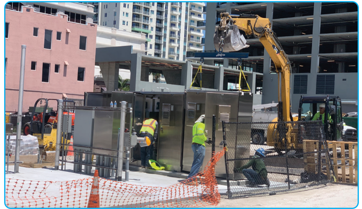
Control panel placement at Pump Station A-7 in Downtown.
