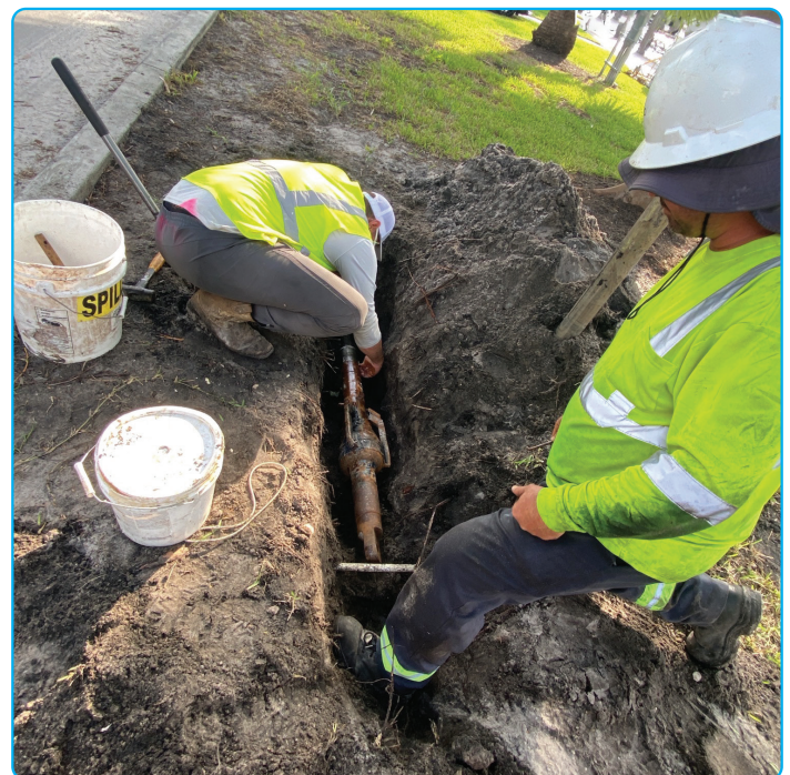
Crews prepare the directional boring machine to pull underground pipe in the Las Olas Isles neighborhood.
