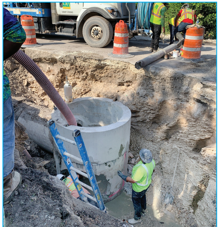
Crews vacuum debris from a new drainage manhole during the installation of a 36-inch concrete pipe.
