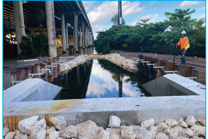
A 72-inch energy dissipater that will protect the New River from erosion is one of the components of the new River Oaks Stormwater System.
