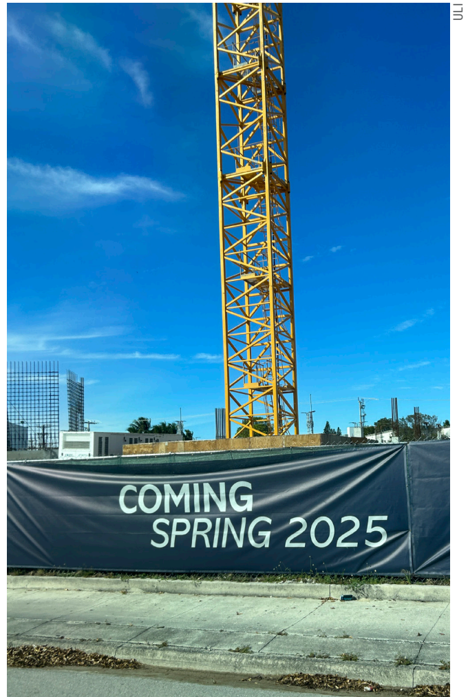
Building cranes around the City are clear signs of the growth that is underway in Fort Lauderdale.
